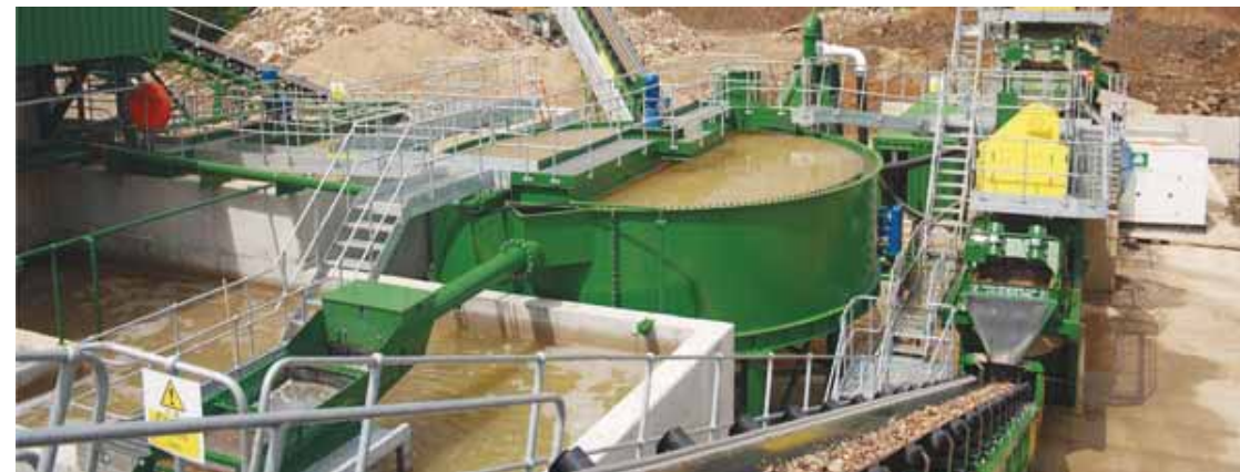
C&D Waste Recycling Plant in Burari
